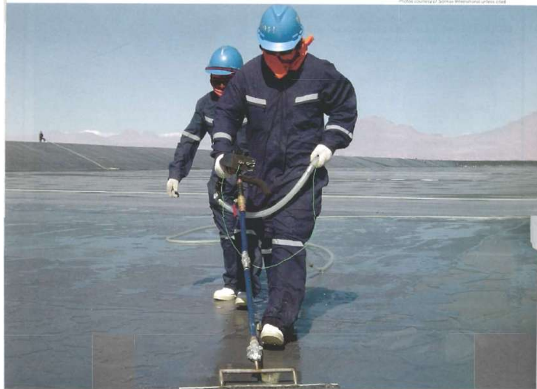
Photo 1 | In constructing the evaporation ponds, after the PVC liner is deployed, electrical leak-detection tests are done (see page 32).
