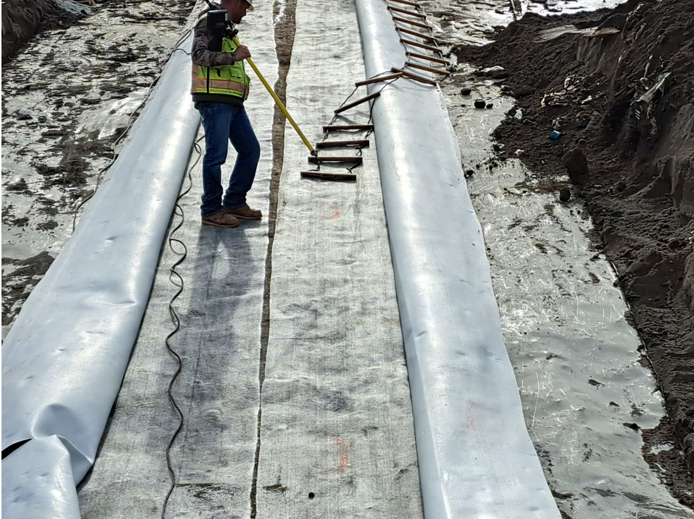
GCL under exposed geomembrane experiencing a gap between adjacent panels; not heat bonded
