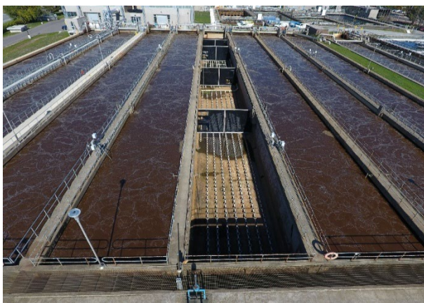
Figure 8. Baffle Curtains for municipal wastewater, Ontario, Canada
