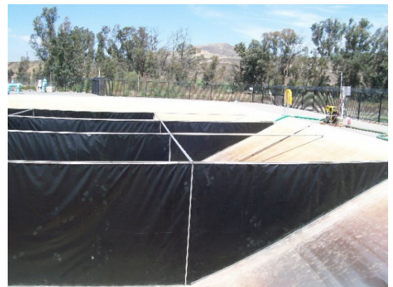
Figure 3. R-EIA baffle curtains for wastewater treatment
