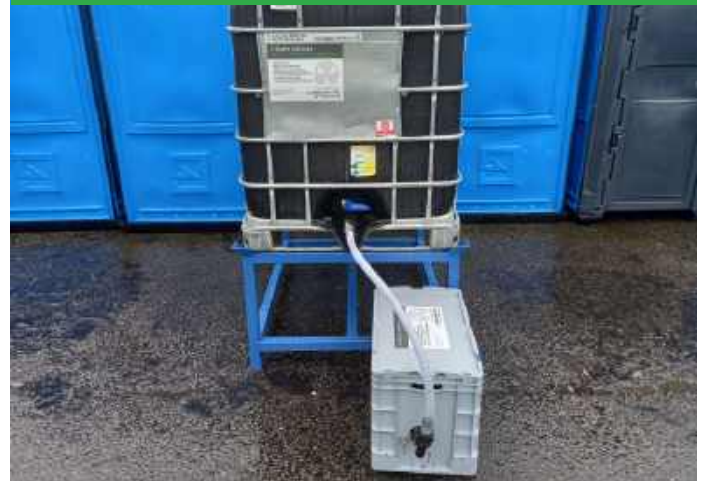
Typical site setup - IBC, pump & protective box
