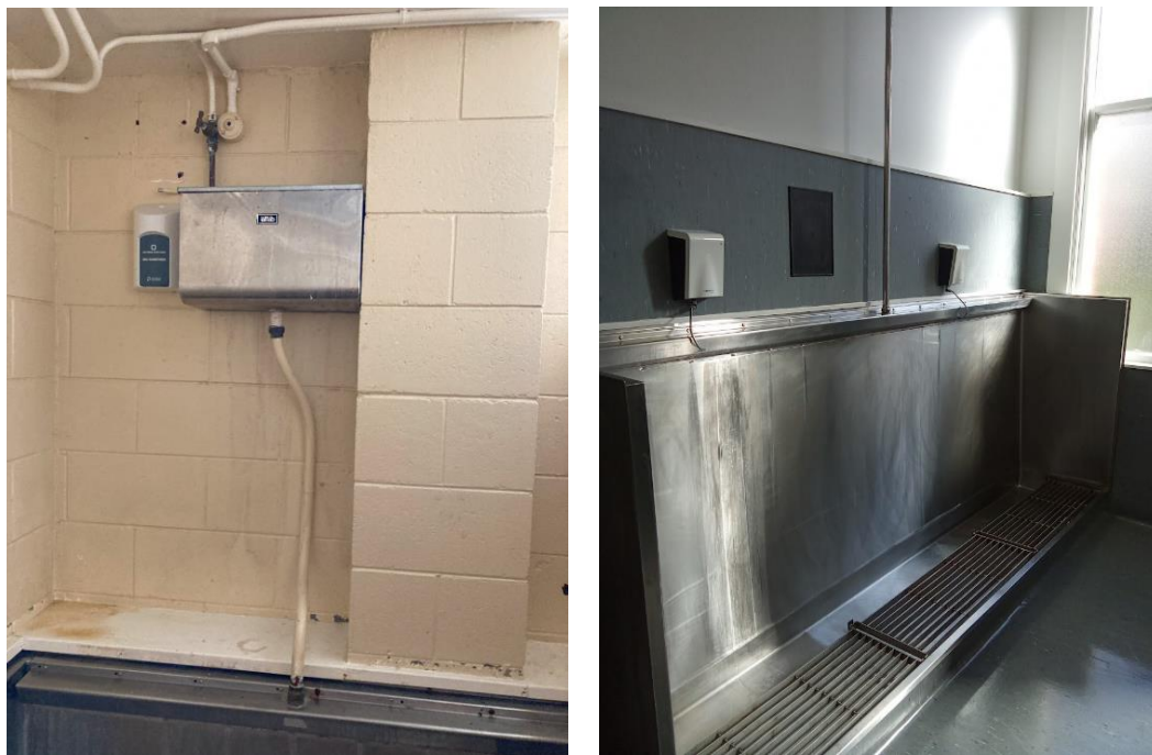
Figure 6 Examples of fill-and-dump urinal tank (left) and tray (right)
