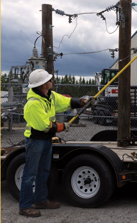
Journeyman Lineworker Blake Huwe performs a high-voltage safety demonstration.
