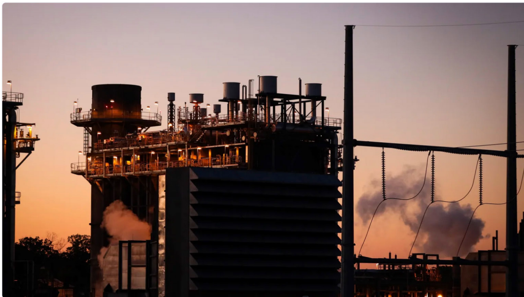
The Potomac Energy Center, a 774-MW natural gas plant located near Data Center Alley in Ashburn, Virginia. The plant was acquired by Blackstone Energy Transition Partners in January. Diana DiGangi/Utility Dive
