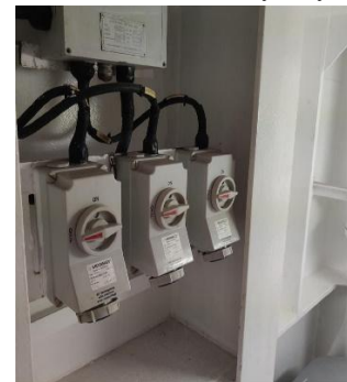
220V SB behind buoyancy-room
