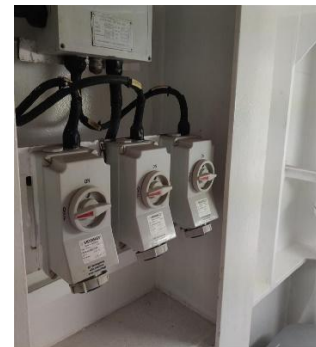
220V SB behind buoyancy-room
