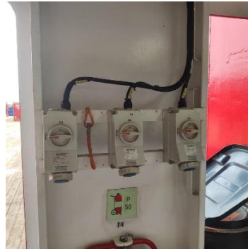
220V PS behind accomodation
