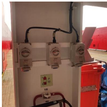
220V SB behind accomodation
