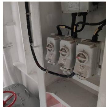
220V PS behind buoyancy-room
