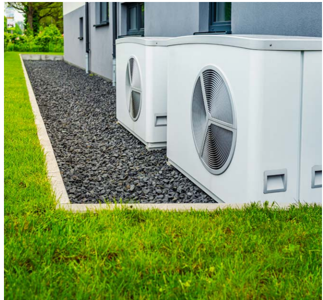
Two air source heat pumps installed outside. Photo credit: Brebca
