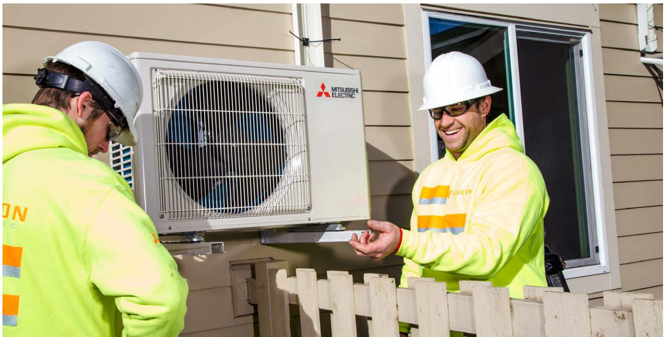
Construction workers install heat pumps in South Seattle, WA. Photo credit: Marcela Gara
