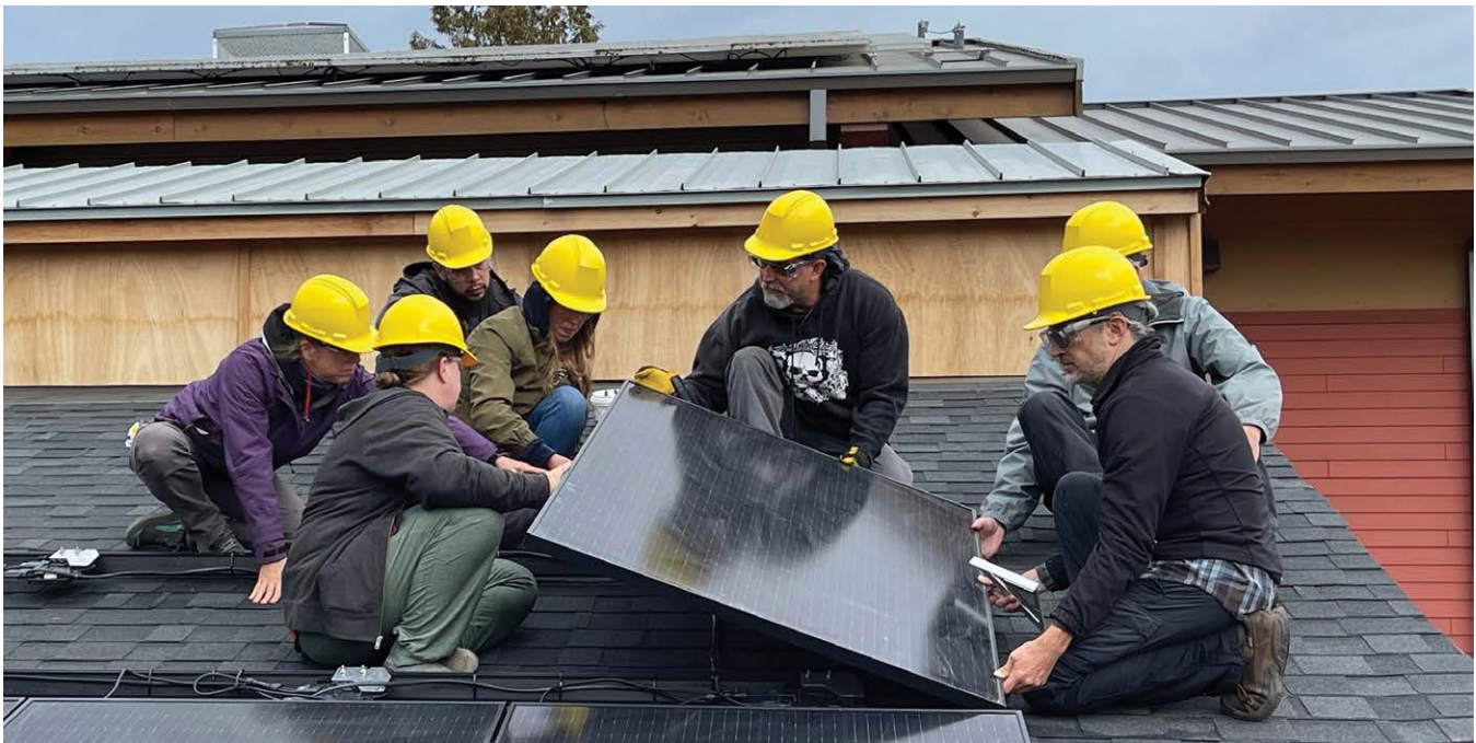
Solar energy technical and vocational training program at the Northwest Indian College, Lummi Nation. Photo credit: Jessica Plumb
