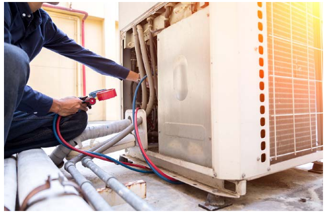
Technician checking air conditioner. Photo credit: A Stockphoto
