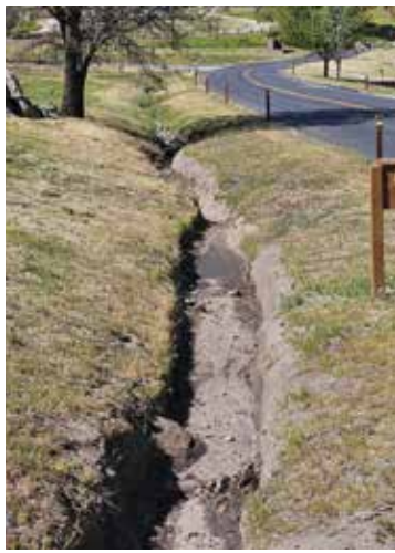
Rolling Oak erosion (before)
