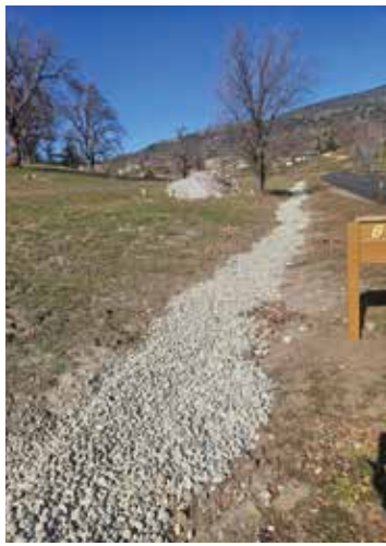
Rolling Oak erosion (after)
