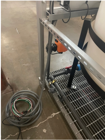
The power whip will be provided to you at the back of the machine. Connect this to your local disconnect.
