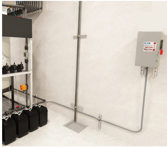
An example of a single batch machine connected to the local disconnect via power whip.
