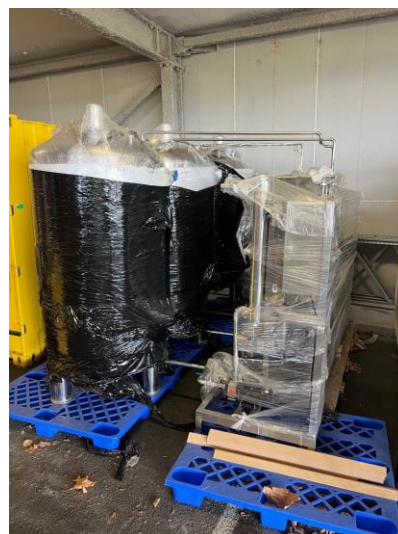
16300s – Reverse Osmosis Plant
