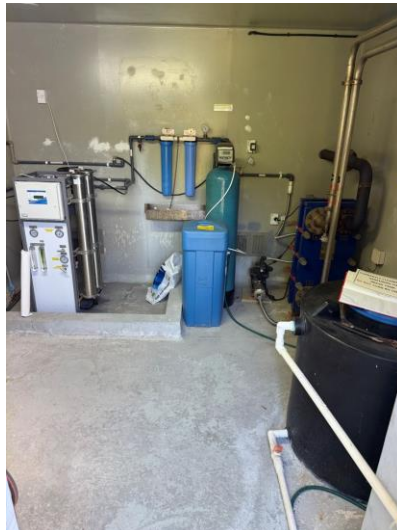
16494s – Reverse Osmosis Plant
