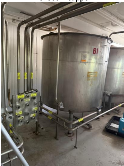
16468s – Tank Farm
