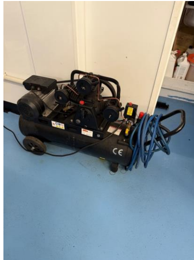
16681s – Air Compressor (x2)
