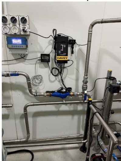
16811s – UV Water System
