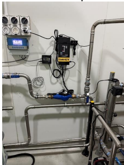
16811s – UV Water System
