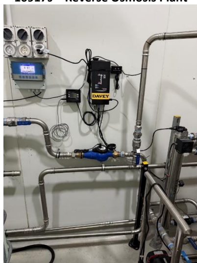
16811s – UV Water System
