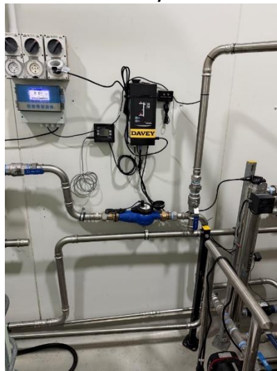
16811s – UV Water System
