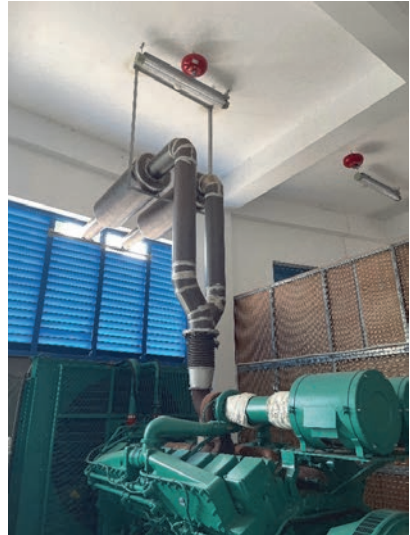
Generator with exhaust and fire sprinkler system, Ever Sun Vietnam 2023
