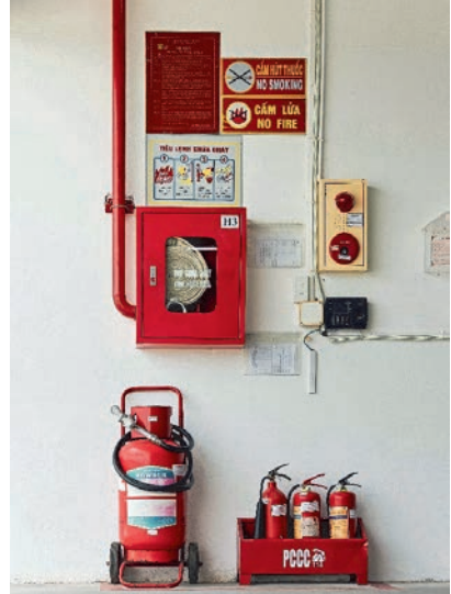
Fire Safety signs, extinguishers and fire hose.Spectre, Vietnam. 2023
