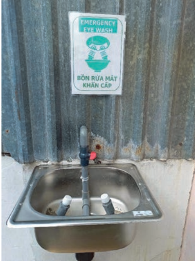
Emergency eye wash station. QVE, Vietnam 2023
