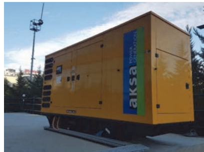
Diesel Generator with complete safety housing.
