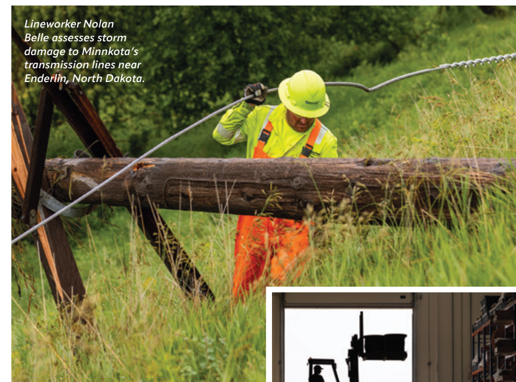
Electrician Mike Howard and Apprentice Electrician Josh Anderson work to repair the Elm River Switch near Hillsboro, North Dakota.
