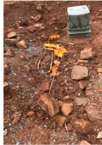
Figure 3: Signaltape Prevented Damage #1
