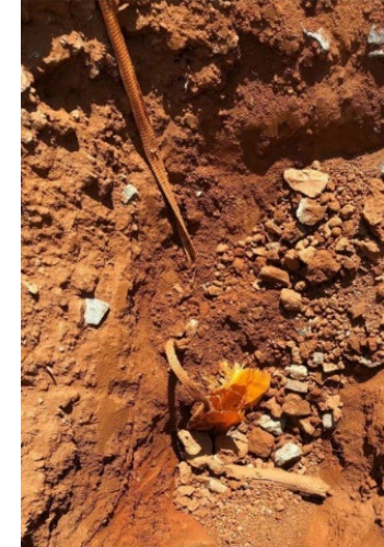
Figure 4: Signaltape Prevented Damage #2
