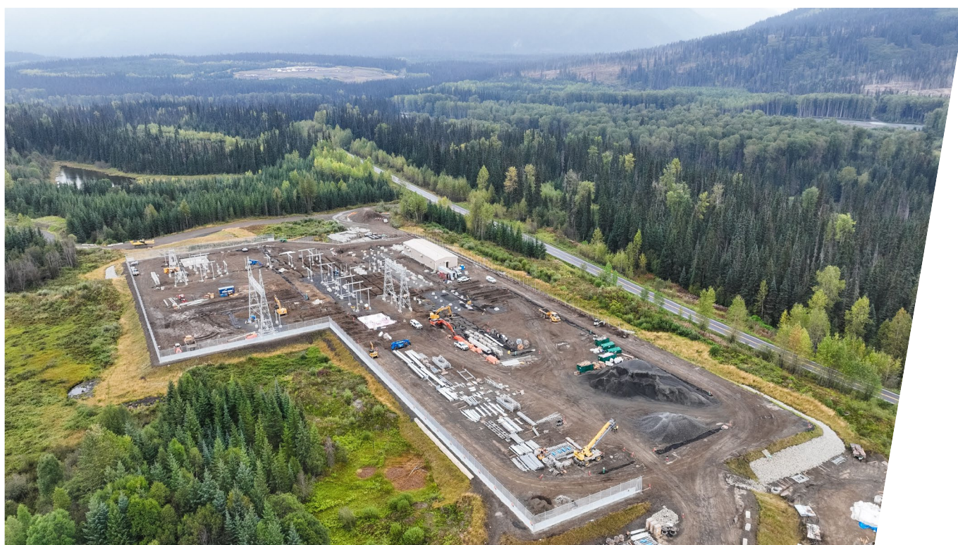
BC Hydro Treaty Creek switching station terminal for power to KSM Project
