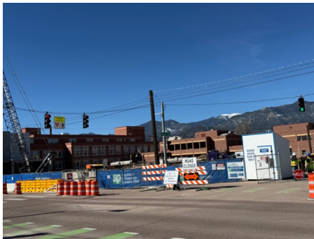
Construction underway at Palmer High School where D11s renovation project prompted important questions about safety, traffic and the future of Boulder Street
