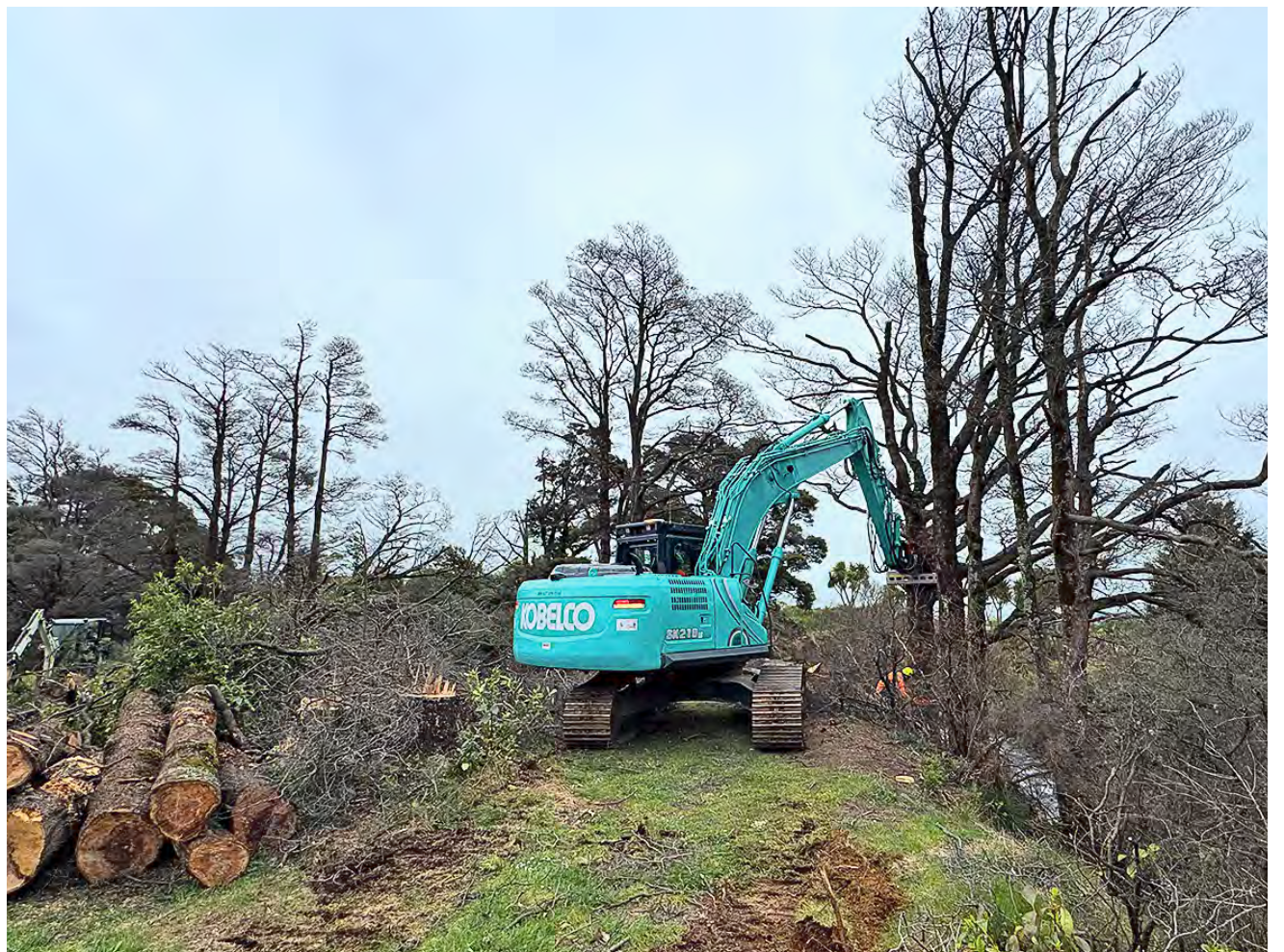
SAD DAY: contractors remove poisoned beech trees from next to the Mangawhero River on Monday. The dead trees were a safety hazard after the criminal damage to around 20 trees.
