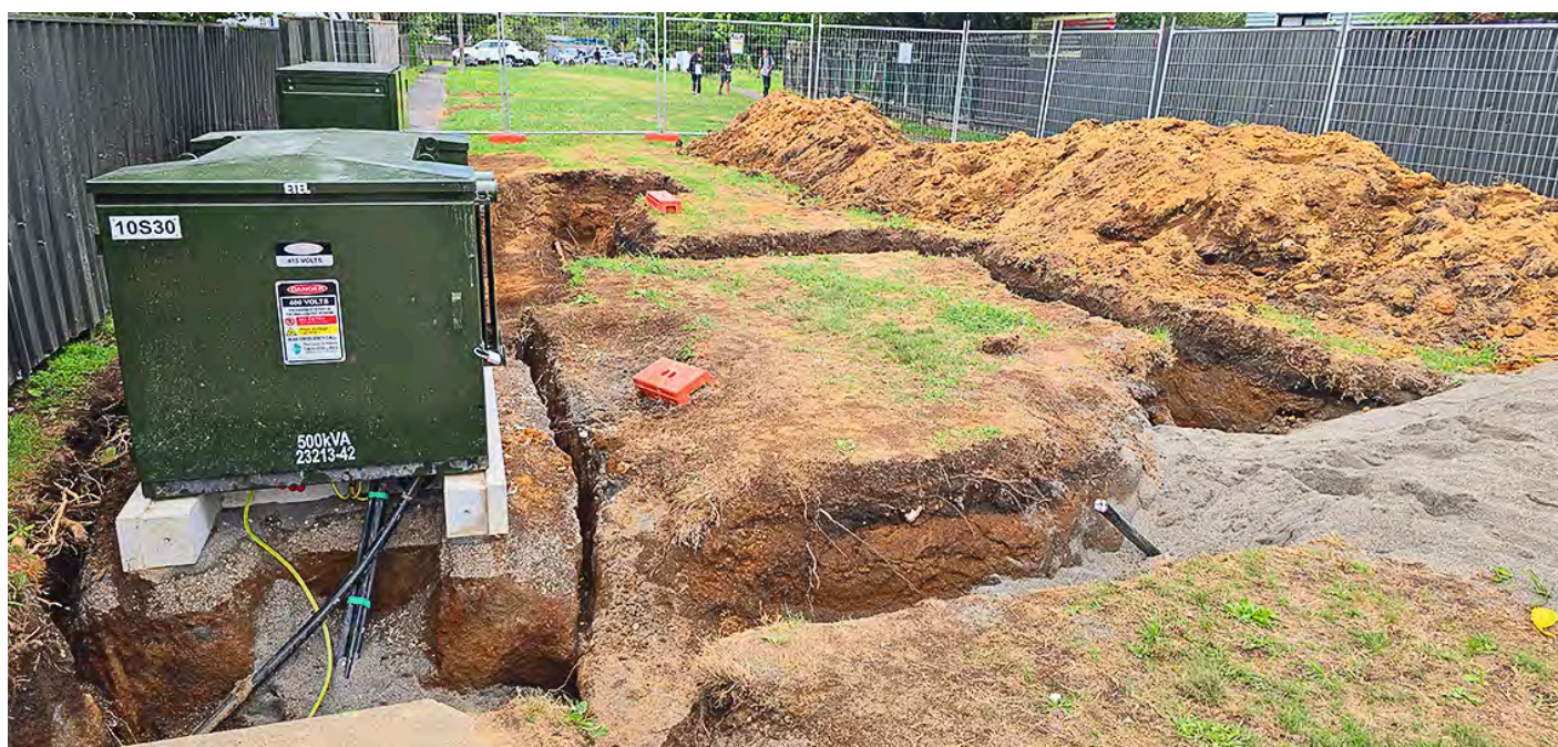
This complex work site takes several weeks to prepare – building concrete plinths and vaults, trenching, installing transformers, laying network cabling, fitting termination kits and other equipment – so it cannot be prepped and completed within a single outage day. That means sites are often left behind security fencing overnight. In the foreground of the photo, a cut aluminium cable (with little scrap value) can be seen protruding from the ground, where it had been connected to the transformer; and additional cabling and termination kits were also stolen from other trenches. Cutting into any buried cable can result in instant death – you cannot tell whether a cable is live just by looking at it. Thieves are putting their lives at risk for very little return.
