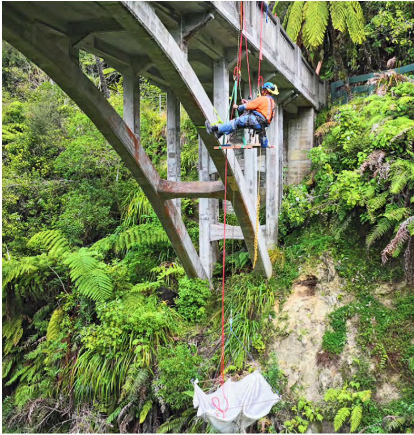
Contractors hang off the side of the Bridge to Nowhere to carry out pre-emptive repairs to lengthen the life of the structure. Photos: DOC.
