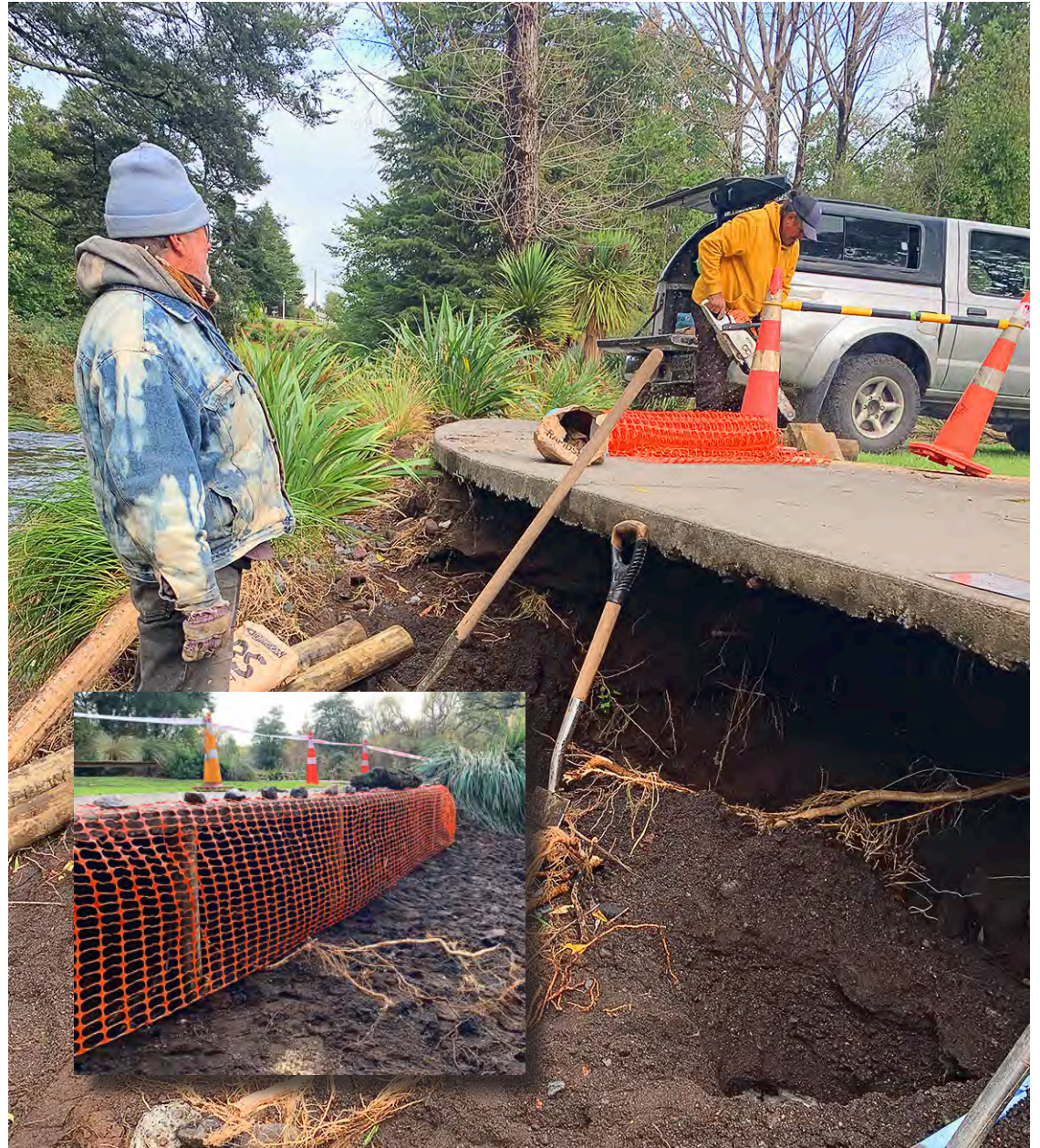
Volunteers Kieran Martin and, at the back Rocky Horne, work on securing a section of the Makotuku Track. Photos: RPCT.
