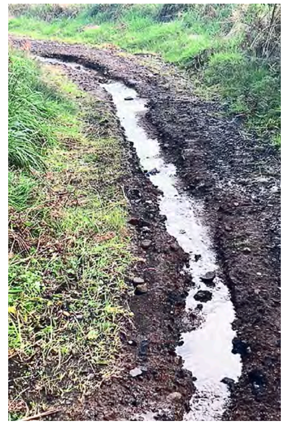
Water damage on Te Ara Mangawhero.
