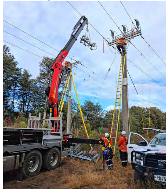
Replacing end-of-life airbreak switch is an integral part of network maintenance to keep our customers connected. Pictured, the team is working on a 33kV line in the National Park area.
