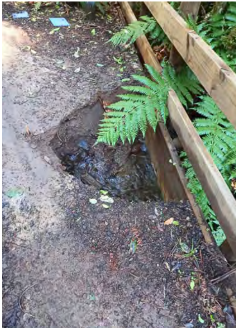
The small hole that was the first sign that something was wrong. Photo: Trevor Taylor.
