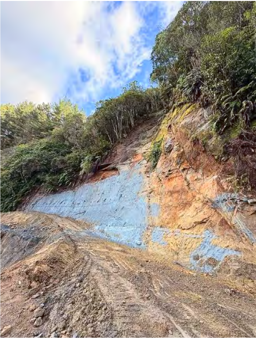
A large slip on Ruatiti Rd in the Ruapehu District was caused by April’s storm.
