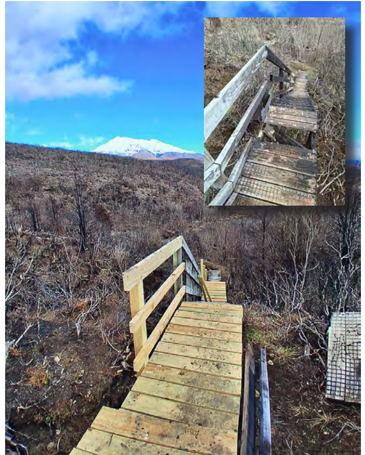
A set of steps after the fire and after the repairs. Photos: DOC.
