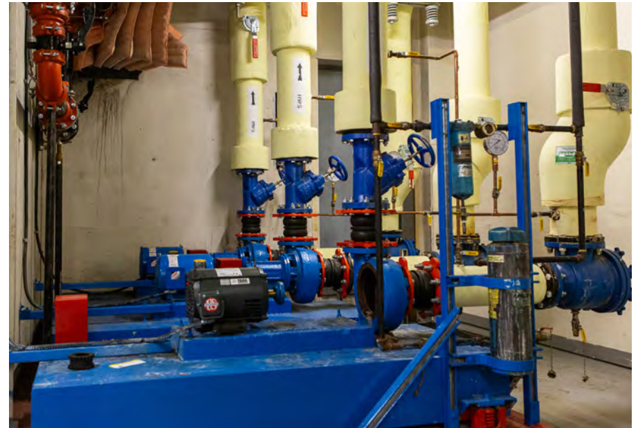
Heating system pumps
