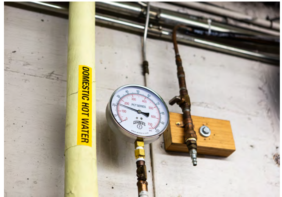
Domestic hot water piping
