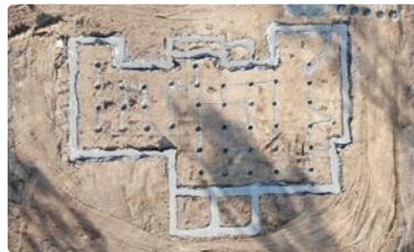
CONVENTIONAL FOOTINGS & SLAB M site with cut/fill to suit* As per plan/spec
