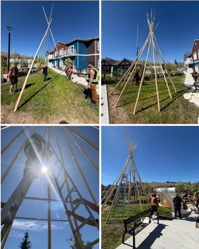
(Top L) Carol Norwegian, Supervisor of Health and Wellness, testing the integrity of three main poles that serve as the backbone for the entire structure
