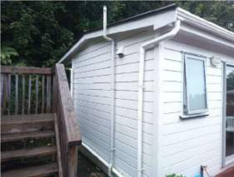
Terminal vent and downpipe outside the ensuite
