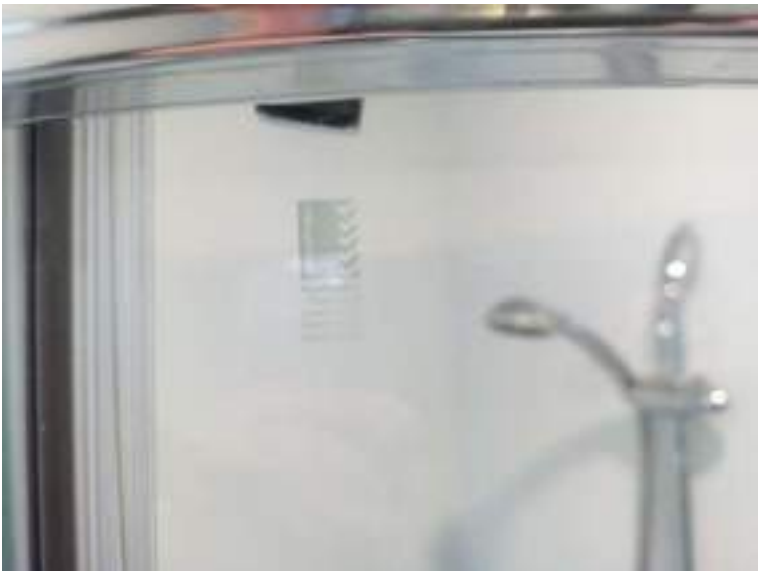
Safety glazing stamp to shower glazing
