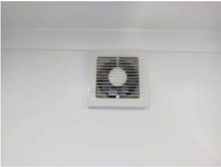
Extractor in the ensuite
