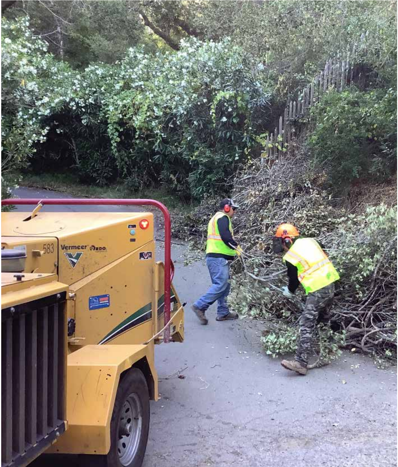
Novato residents take advantage of Marin Wildfire's Chipper Program to remove vegetation.
