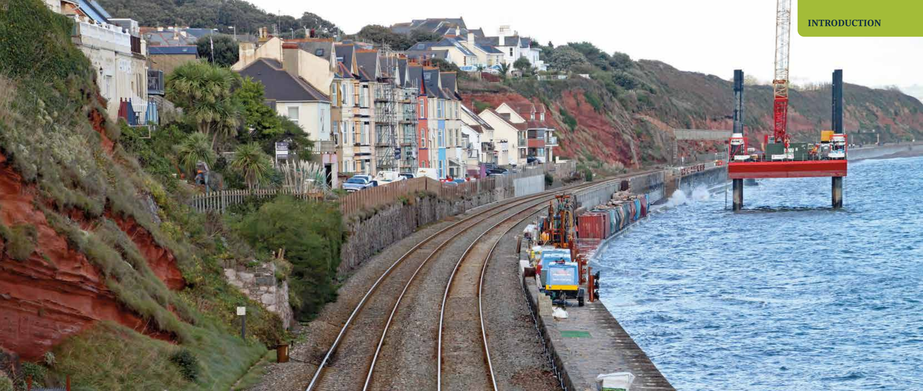
▲ Repair works at Dawlish railway station following the collapse of the tracks during storms in 2014. © Anthony | Adobe Stock
