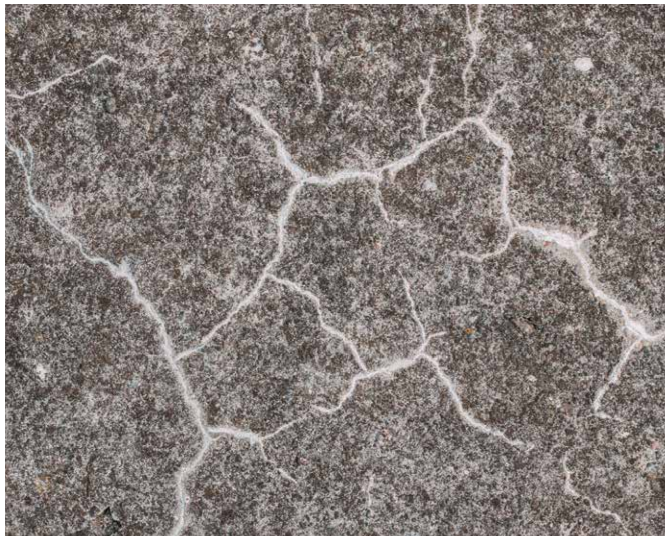
▲ Concrete with bacteria-healed cracks. © photosvideos | Adobe Stock
