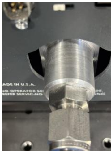
Figure 5: Properly installed VCO vacuum line
