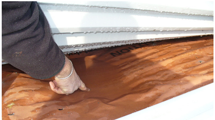
Figure 9: Ponding of a membrane installed in NZ at extremely low pitch with no rigid support board or structured ventilation strategy.
