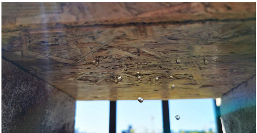
Figure 10: Water dripping through a vapour permeable Oriented Strand Board (OSB 3 type product). This is an ideal vapour permeable solution for supporting the membranes but cannot be used for waterproofing by themselves.
