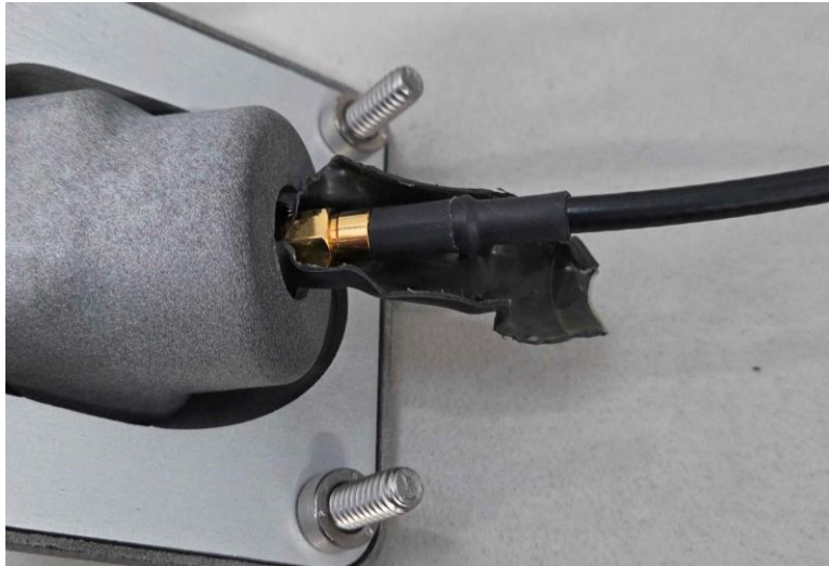
Figure 39 Heat shrink partially removed, SMA junction exposed
