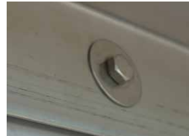
Close up of bolt through washer and mounting angle
