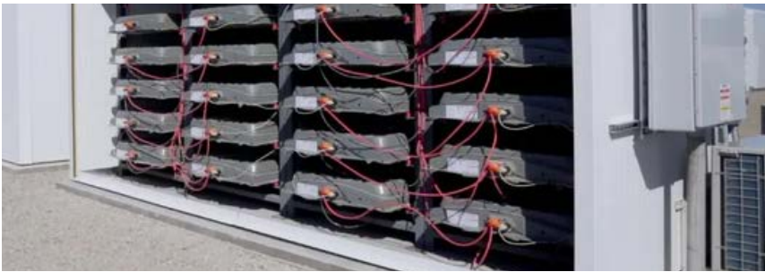
Figure 5c: EV Battery Storage System
