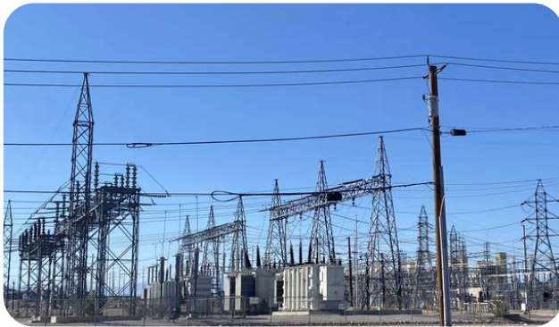
Figure 3: NV Energy's Clark Generating Station in Henderson
