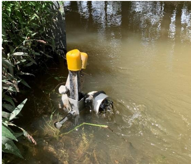
Figure 4: Installed tile drainage flow meters enabled flow data capture on sites where the receiving water body regularly submerged the tile exit, therefore inhibiting manual flow data collection during monitoring runs. This allowed more regular data capture at these sites.
