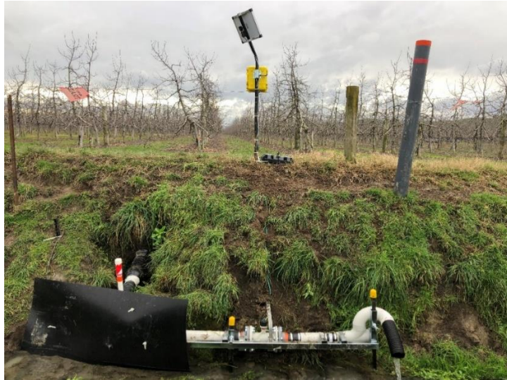
Figure 3: Tile drainage flow meter equipment, installed at a monitoring site, allowing for continuous flow data capture
