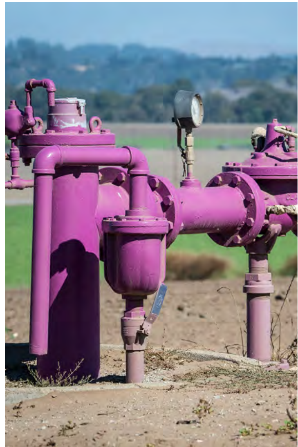
Purple pipes for water reuse © Lance Cheung / USDA
