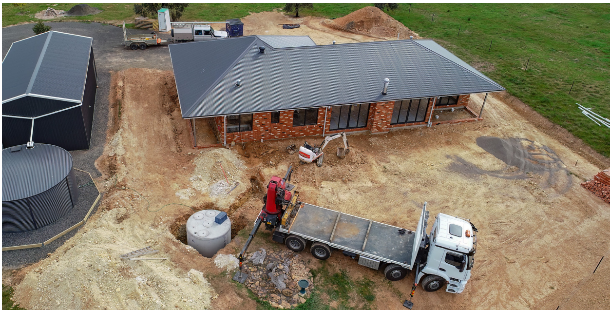
Septic instal © royalty free
