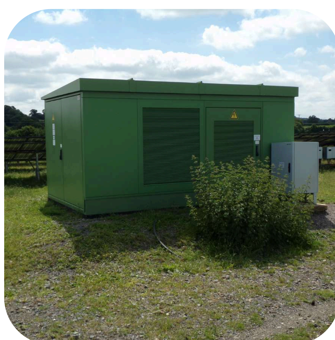
Transformers and storage containers
