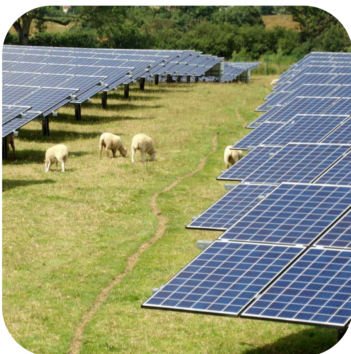
Fixed tilt PV panels
