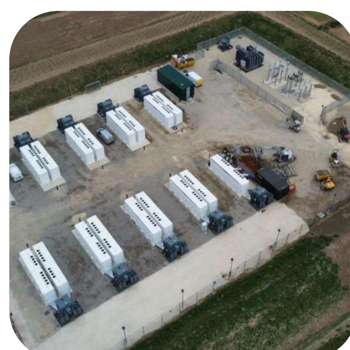
Battery storage units for load shifting / flexibility services
