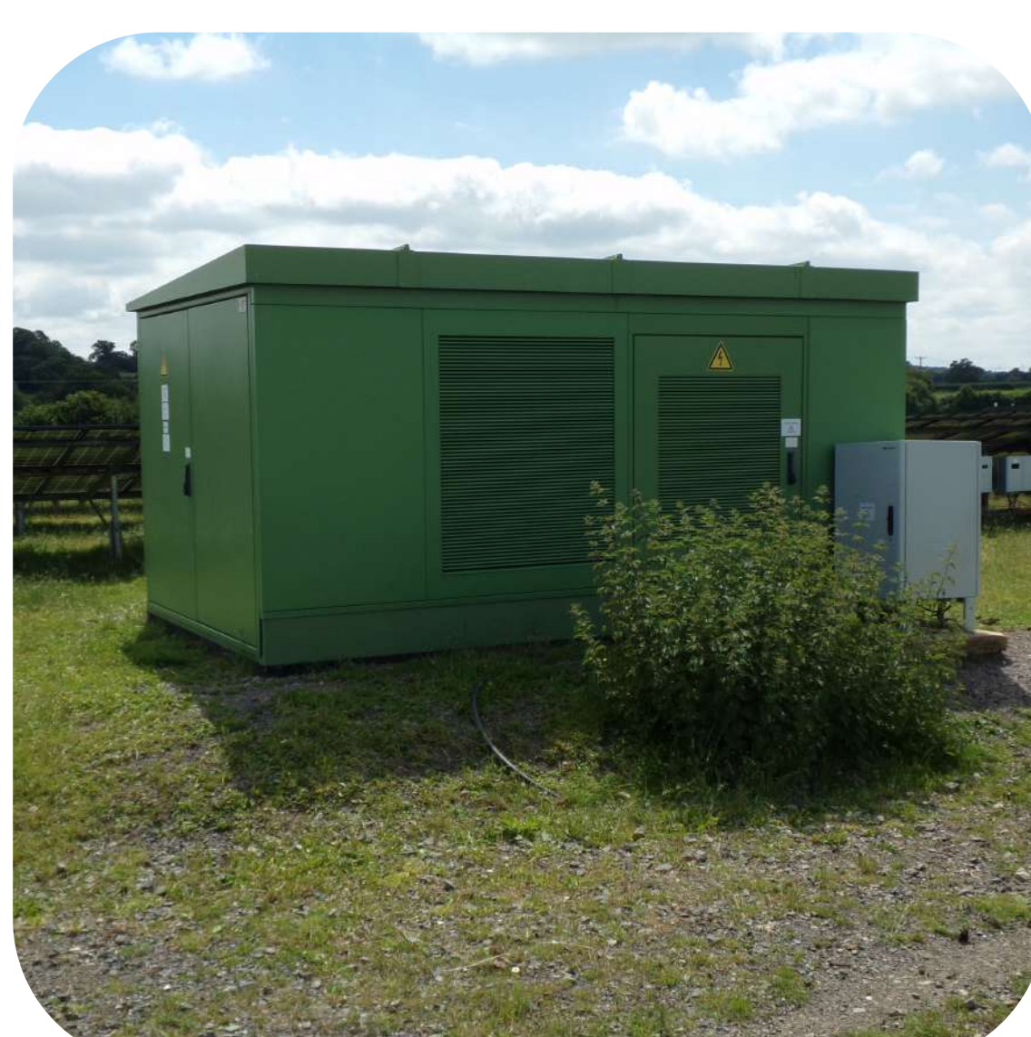
Transformers and storage containers
